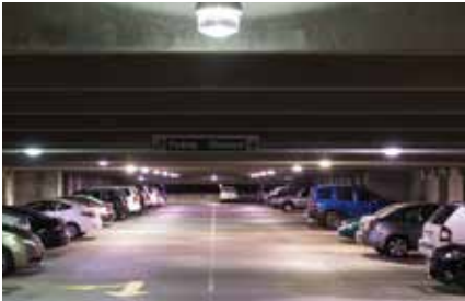
Before: Metal Halide Lighting
