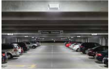
After: Cree WaveMax® Technology LED Lighting
